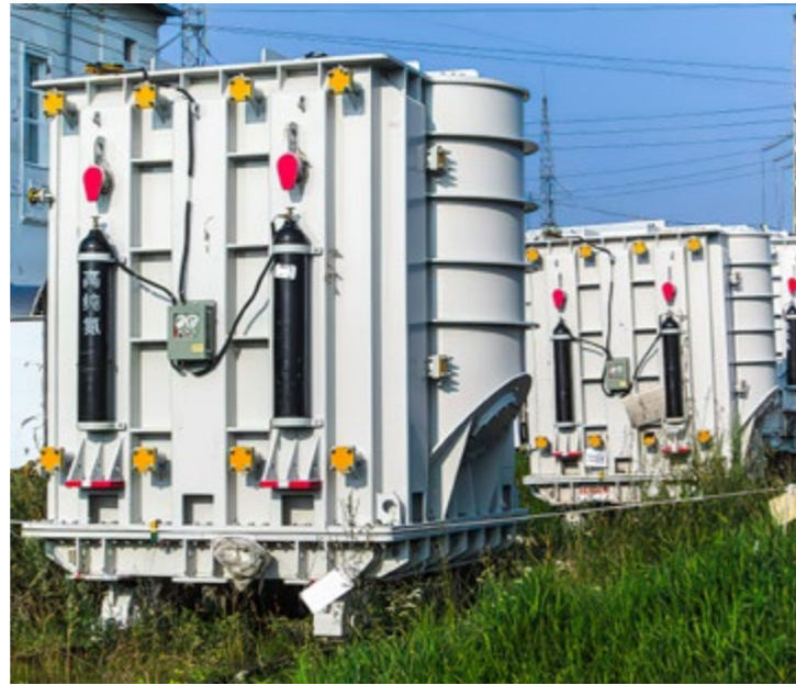
▲ 60MVar/500kV Shunt Reactor Tulum Substation, Russia
