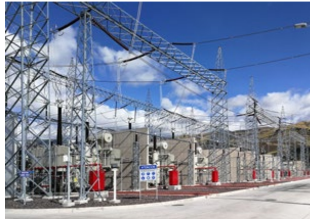
▲ 250MVA-500kV Transformer Inga Substation Ecuador
