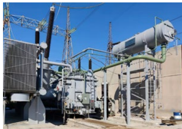
▲ 280MVA-400kV Transformer Koumoundourou Substation Greece
