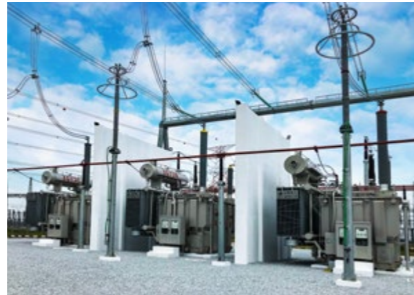
▲ 350MVA-500kV transformer Olak substation Malaysia
