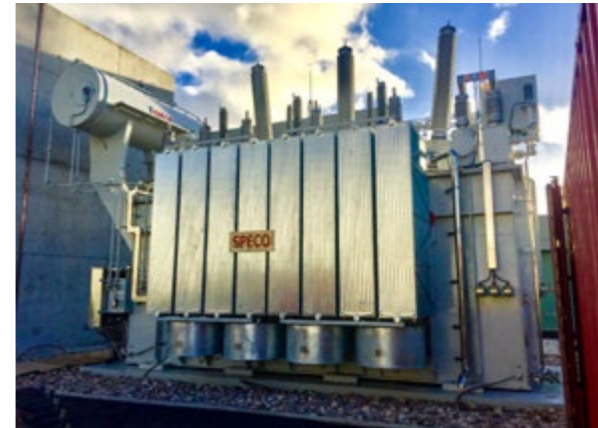
▲ 170MVA-220kV Transformer Carregado Substation, Portugal
