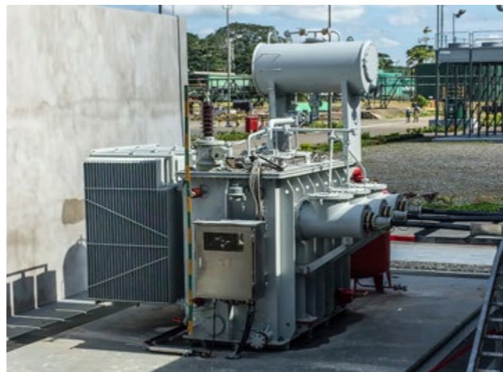
▲ 50MVar/66kV Shunt Reactor Ecuador
