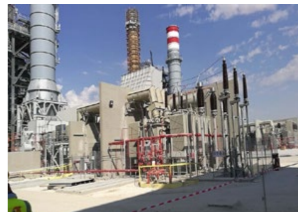
▲ 220MVA-132kV Transformer Hussein Power Plant Jordan
