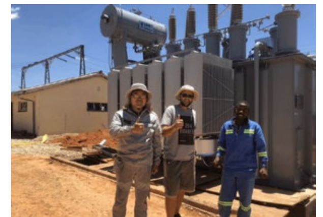
▲ 50MVA-132kV Transformer Nyanga Substation Zimbabwe
