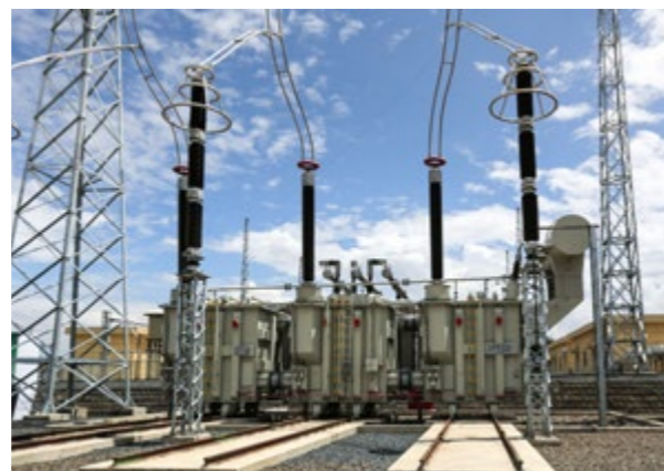
▲ 315MVA-400kV Transformer Holeta Substation Ethiopia
